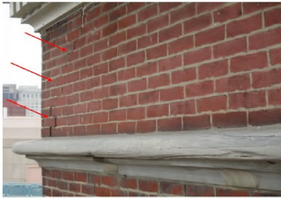
Cracking & repointing of brickwork
