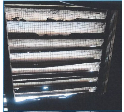
Deteriorated Steeple Louvers
